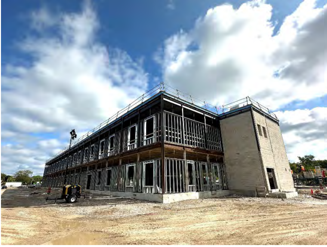
The 550 pupil new North Shore school located in Tecumseh is just down the street from D.M. Eagle PS. It has a large play space outdoors with a beautiful double gym. A large library exists off the entrance and the school has a number of child care rooms. The students will be moving into a bright 21 st century learning environment.
